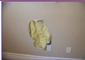
Damaged area at wall
