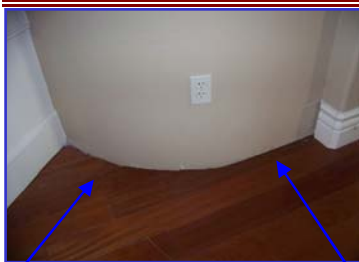
Missing base board at entry
