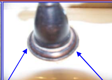
Evidence of previous leak around faucet@ right sink
