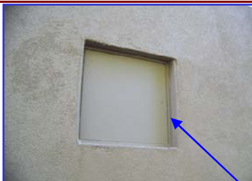
Access door under tub.could not be opened
